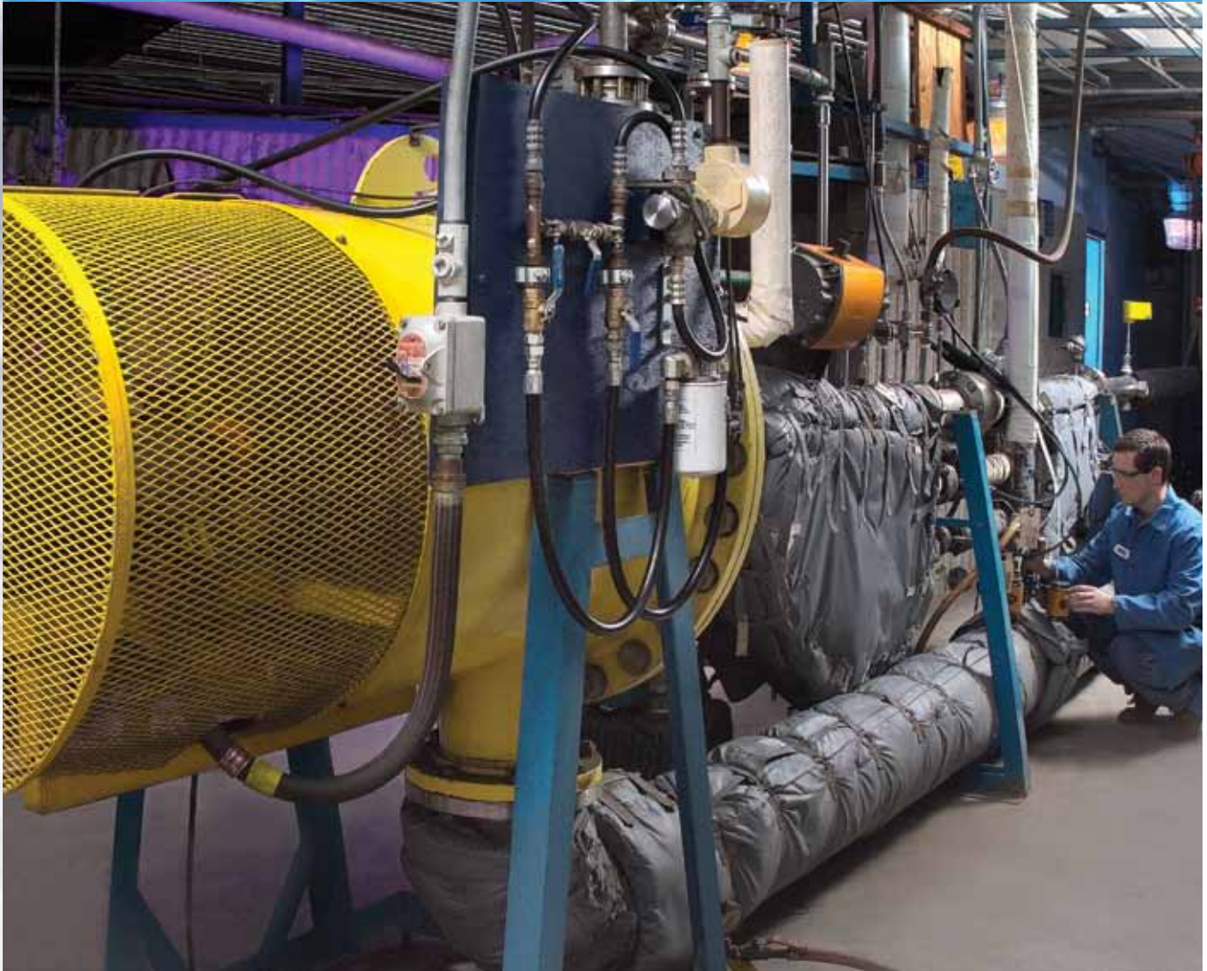
Pressurized gas loop stand
