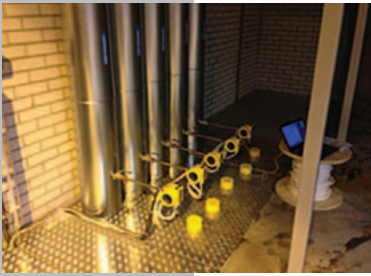
FCI ST100 in wastewater treatment plant
