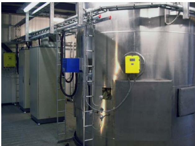
Figure 3. Installed MT91 Flow Meter
