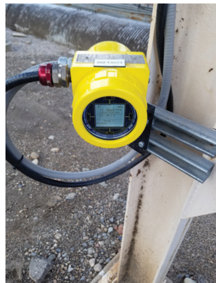
Figure 2: Installed ST100 Flow Meter
