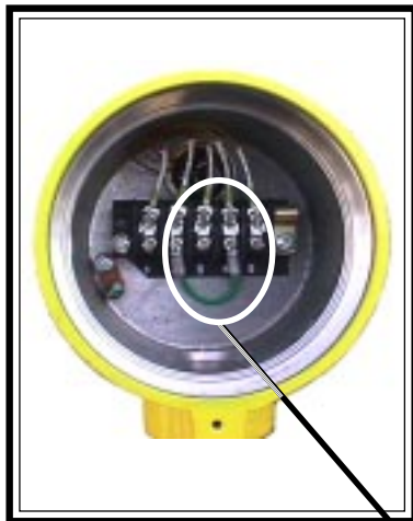
Flow Element Wiring Diagram (Be sure the jumper is in place Terminal 2 to terminal 4.)
