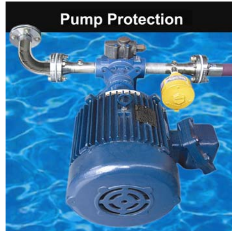
Fig 1. Pump with Flow Switch
