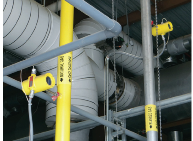
Installed FCI Model ST98 thermal mass flow meters.
