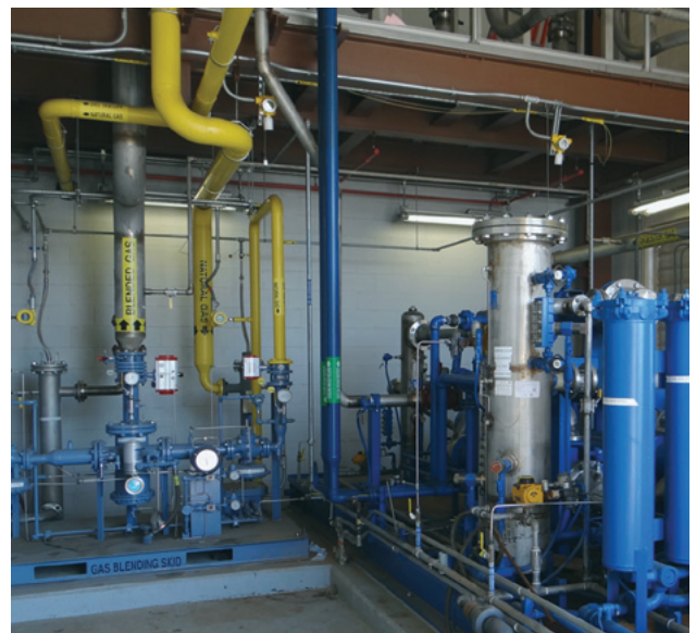
Blended waste gas and natural gas system is used to operate a New Jersey facility's co-gen engines.
