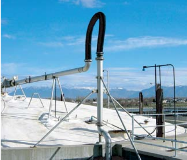
Figure 1. Typical wastewater treatment digester gas bag system.
