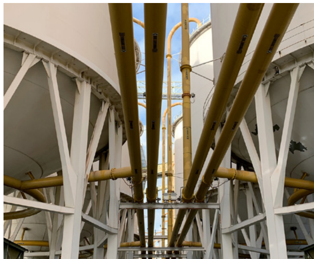
Figure 1: Silos with fumigant piping
