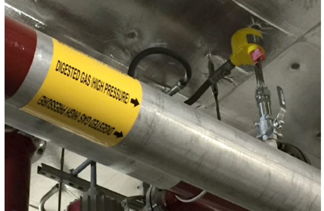
Figure 3: Installed ST80 flow meter in co-gen building
