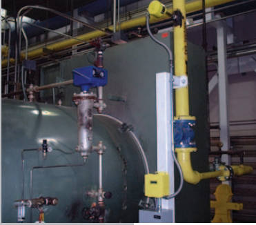
Boiler with FCI ST98 flow meter
