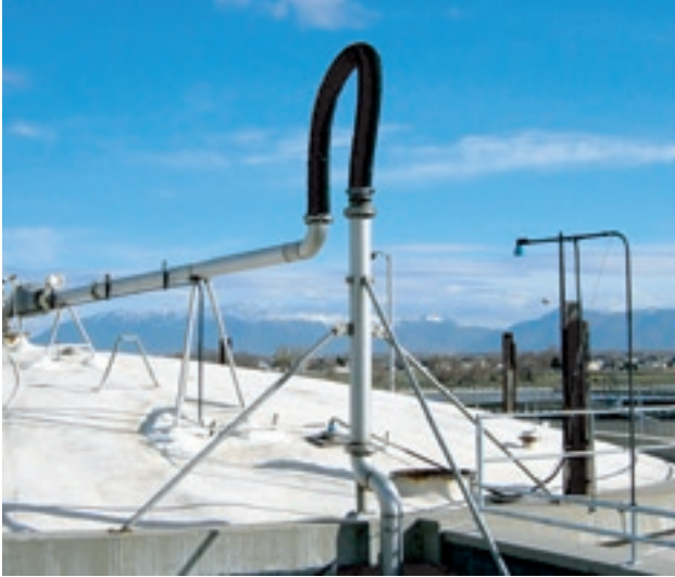
Figure 1. Typical wastewater treatment digester gas bag system.
