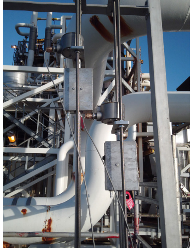
Figure 4: Installed thermal flow meter on flare gas vent line
