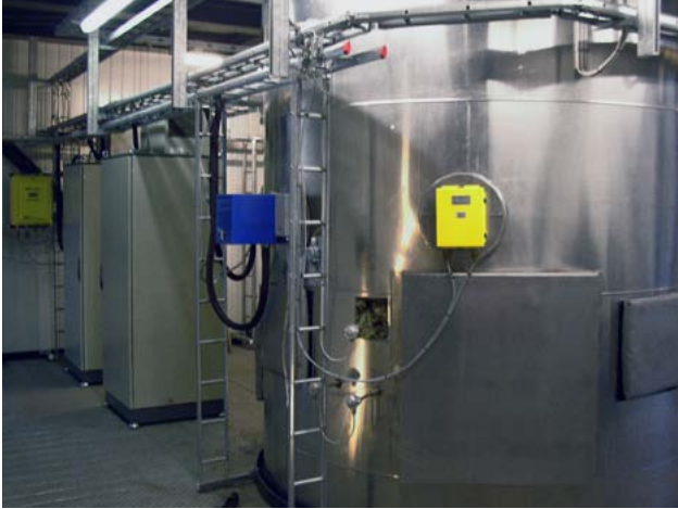
Figure 3. Installed MT91 Flow Meter
