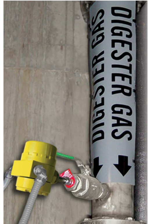
Figure 5: Flow meter installed on digester gas pipeline
