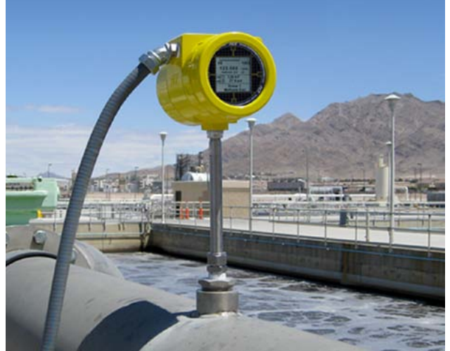
FCI ST100 Series Flow Meter at WWTP trial site
