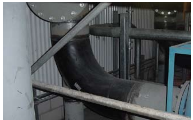
Figure 4. Electric Power Plant Elbow and Pump
