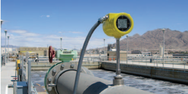
Figure 1. FCI ST100 Thermal Flow Meter at WWT Plant
