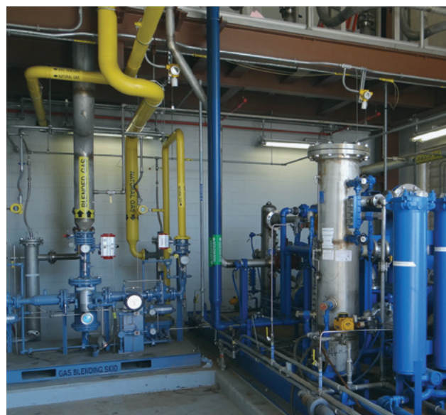
Blended waste gas and natural gas system is used to operate a New Jersey facility's co-gen engines.
