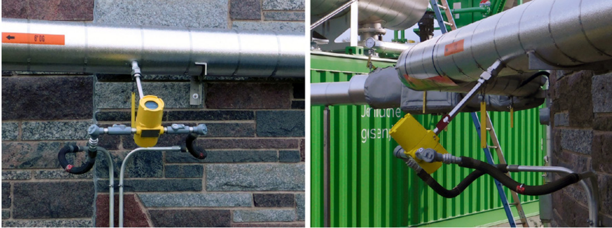
Figure 4: FCI Model ST98 installations
