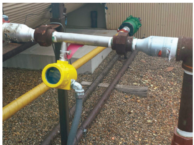
Figure 3: FCI Model ST75V flow meter installed at well head
