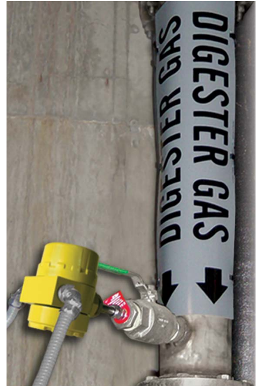
Figure 5: Flow meter installed on digester gas pipeline
