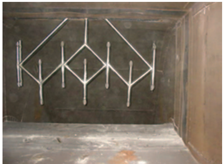
Figure 4: Averaging pitot tube flow meter in primary air duct
